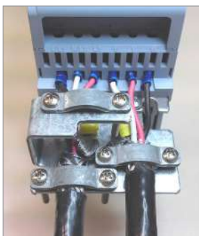
Figure 3.3: Details of the connection of the power supply and the motor cable shield to the accessory CFW500-KPCSA
